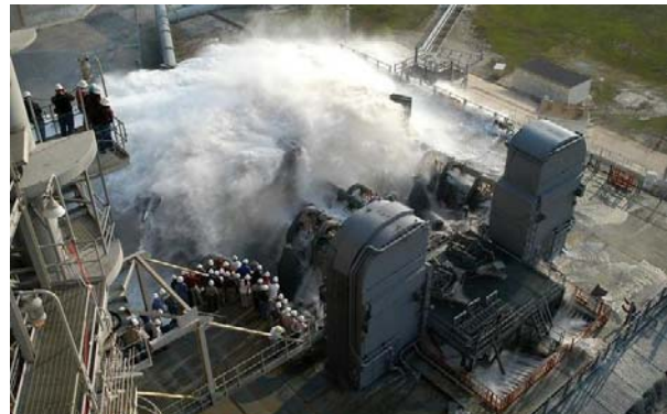
Sound Suppression System test on launch pad 39A at the Kennedy Space Center. (Image: NASA)
